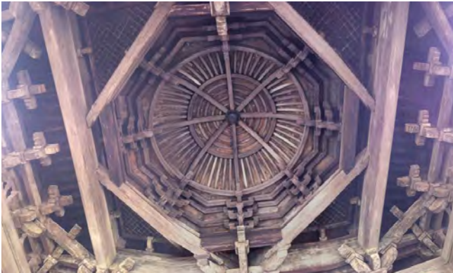
Fig. 4. Jinci temple, Shanxi province, built 1023-1032 CE, Song Dynasty corbels and post and lintel roof structure. Image, Hursty.
